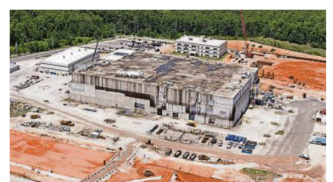
Savannah River Site opens new construction fronts to build its plutonium facility.
